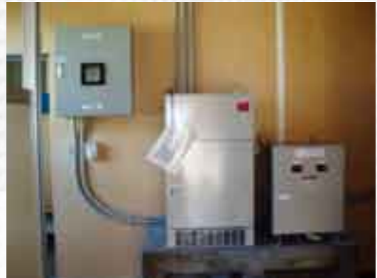
Protecting device, power conditioner, transformer
